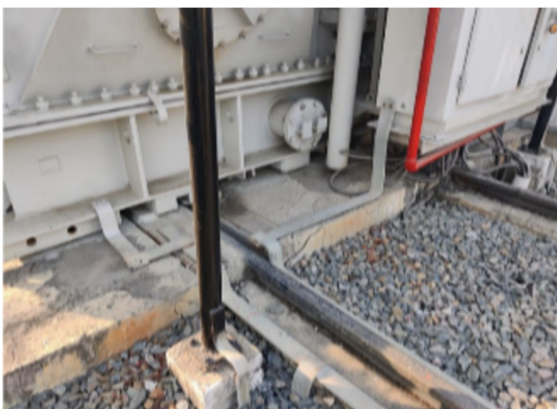
Fig. 1. Reactor foundation, front view with cracks.
