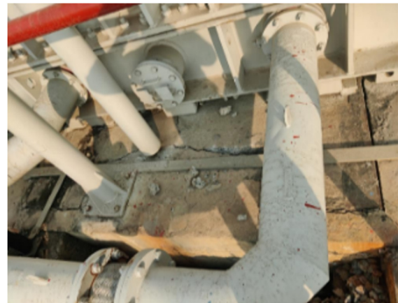
Fig. 2. Reactor foundation, back view with cracks.
