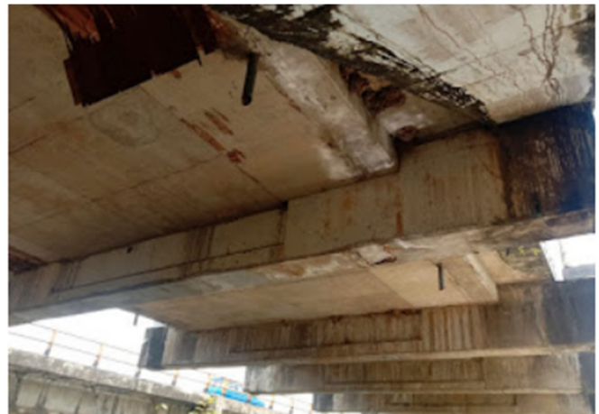
Fig. 1. Existing failure conditions of the Pute Bridge-river deck slab. Surface cracking, concrete spalling, and localized deterioration were observed during the field inspection.
